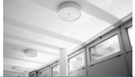
Fig. 11: Light redirected by special glazing in the upper windows of the library
