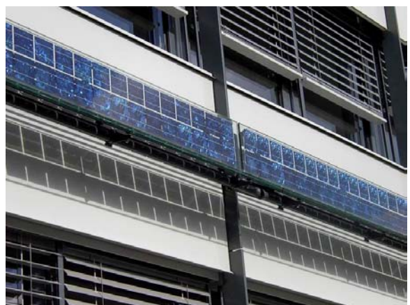
Figure 16: view on the lower pair of modules with no visible mounting member.
