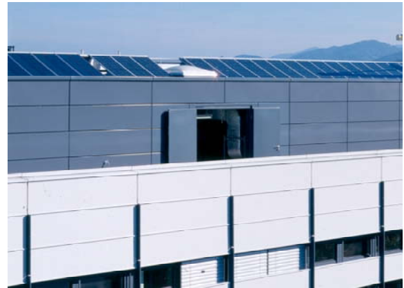
Figure 4: The PV generator on the flat roof of building C. At the left side test modules can be seen, which will be replaced in November 2001 (photo: Guido Kirsch).
