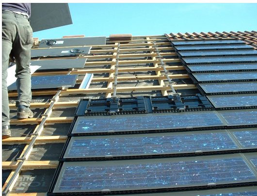
Plastic tray installed with PV module about to be placed on it
