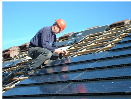
Making the electrical connections using the straight forward Multi-Contact plug system
