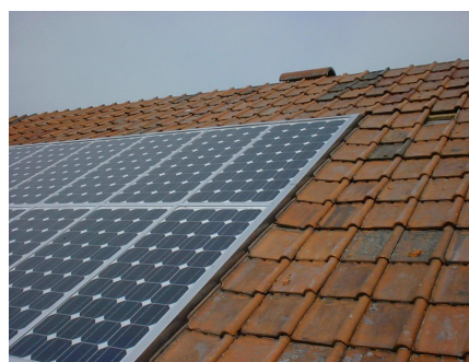
The completed PV array
